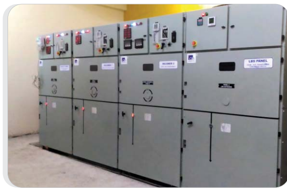
33kV VCB Panel
