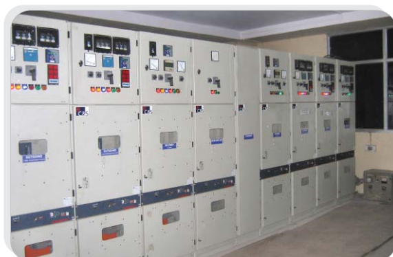
11kV VCB Panel
