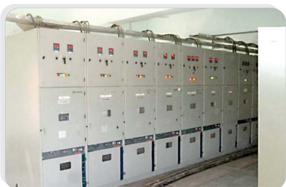
22kV VCB Panel
